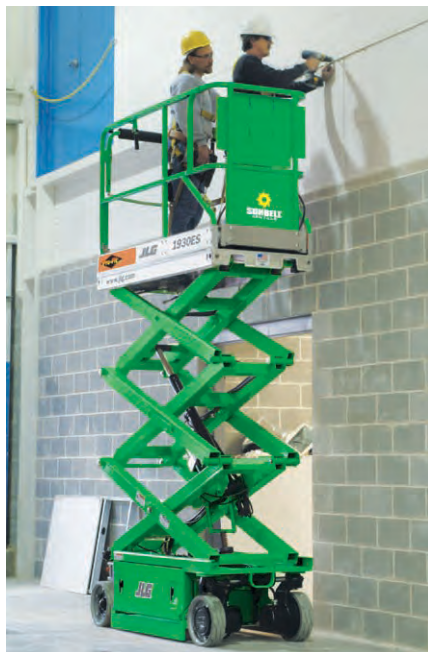
▲ Sunbelt Rentals is one of the largest equipment rental companies in North America, with more than 825 locations.
